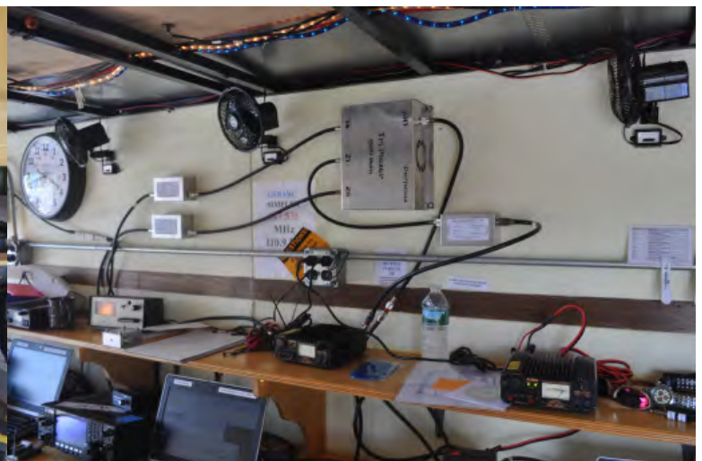
The Triplexer for the CW stations
